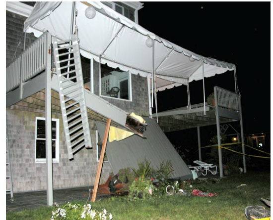
Ten partygoers were injured when this deck on Martha’s Vineyard collapsed in August 2003.
