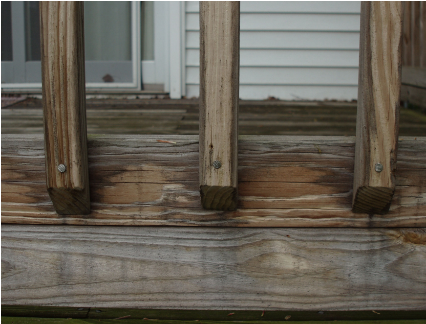
An adult falling into this railing could easily cause it to pull away from the deck, causing an accident.
